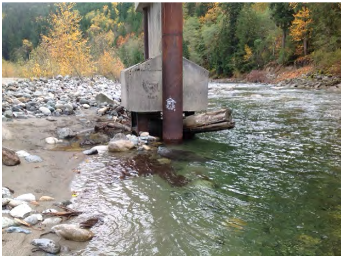
log under pier 2
