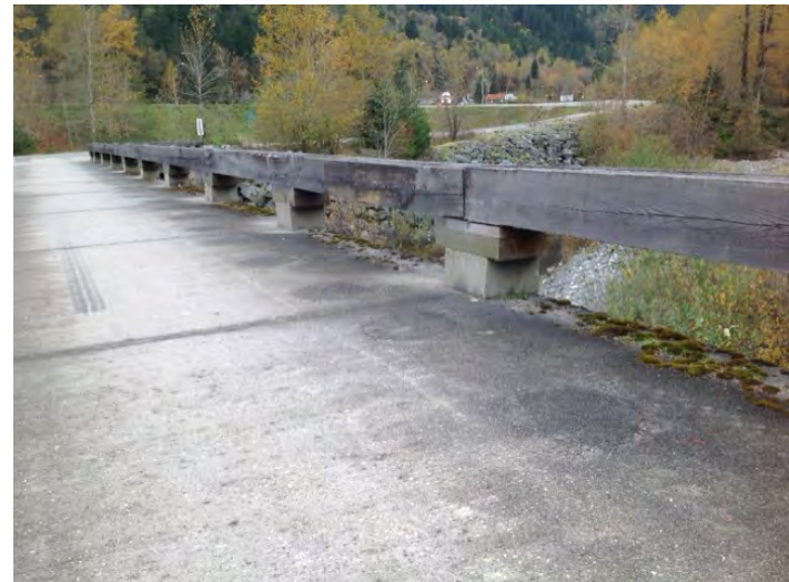
Guardrail on span 3
