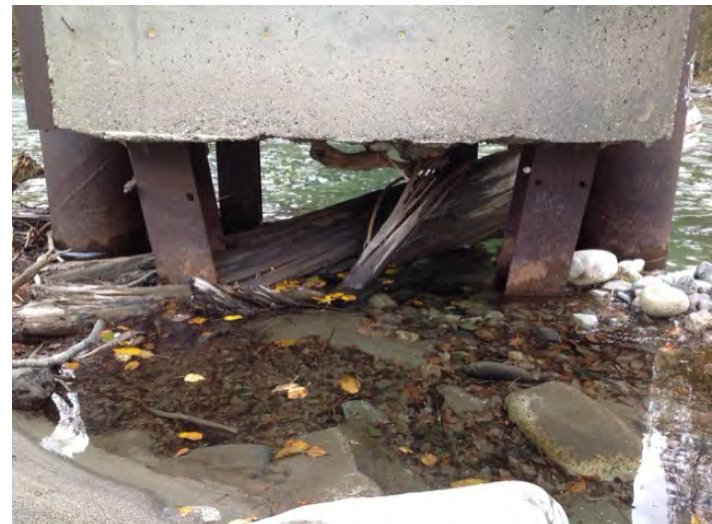
log under pier 2
