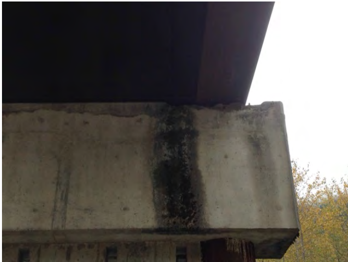
pier 2 spalling concrete
