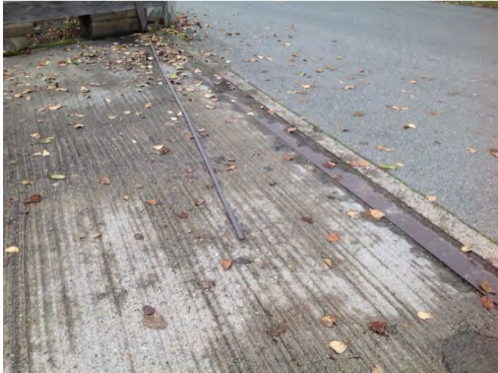
steel separation on span 3 at road surface
